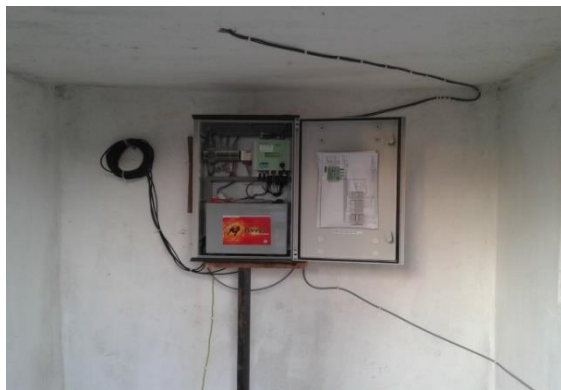
Example of a data logger housing fixed on the wall
