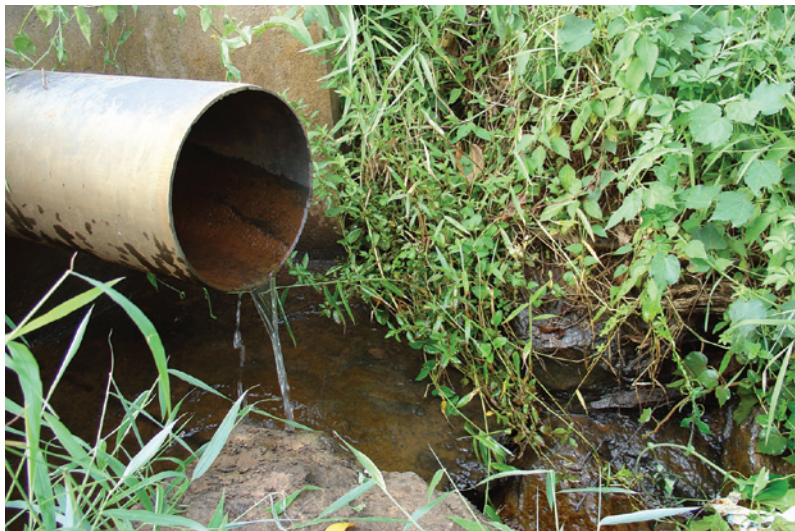
The monitoring and control of effluent flowing into water bodies is one of WRMA's core functions.
