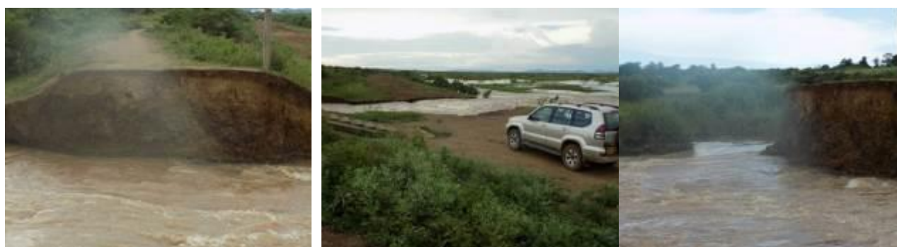
Figure 3.13: Flooding in Lower Nzoia: Left -Breached Dyke at Dominion. Middle -Flood flow into the farms. Right - Diverted river flow
